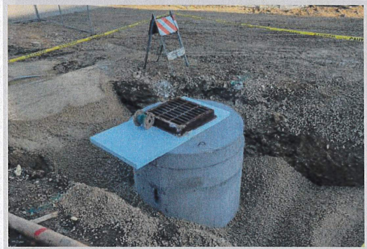
Above: Last storm structure installed in the parking lot area and tied into Mayville Storm Sewer system.
